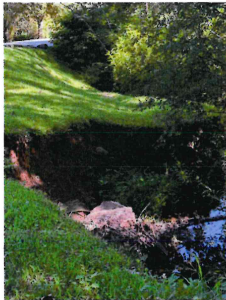
Existing Erosion at Lot ID 6
